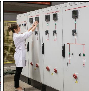
SMART GRID AND DISTRIBUTED GENERATION LAB
